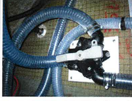
MANUAL PUMPS TECHNICAL ROOM
