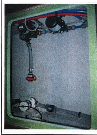
AFT STARBOARD GANGWAY BILGE PUMP
